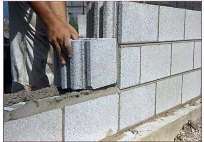
Fig. 4. Avoid spreading mortar too far ahead of units. Place unit on mortar bed as quickly as possible. (IMG13631)
